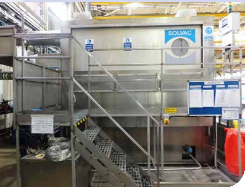
Bespoke Solvac Cleaning System installed at BAE site in Brough
