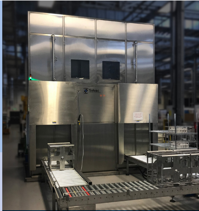
Bespoke Solvac TA machine installed into West Midlands Aerospace manufacturers facilities by Fraser Technologies.
